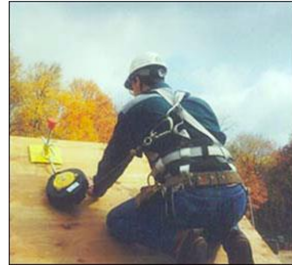
Photo: Figure 13: OSHA Guidance doc on fall protection in residential construction
